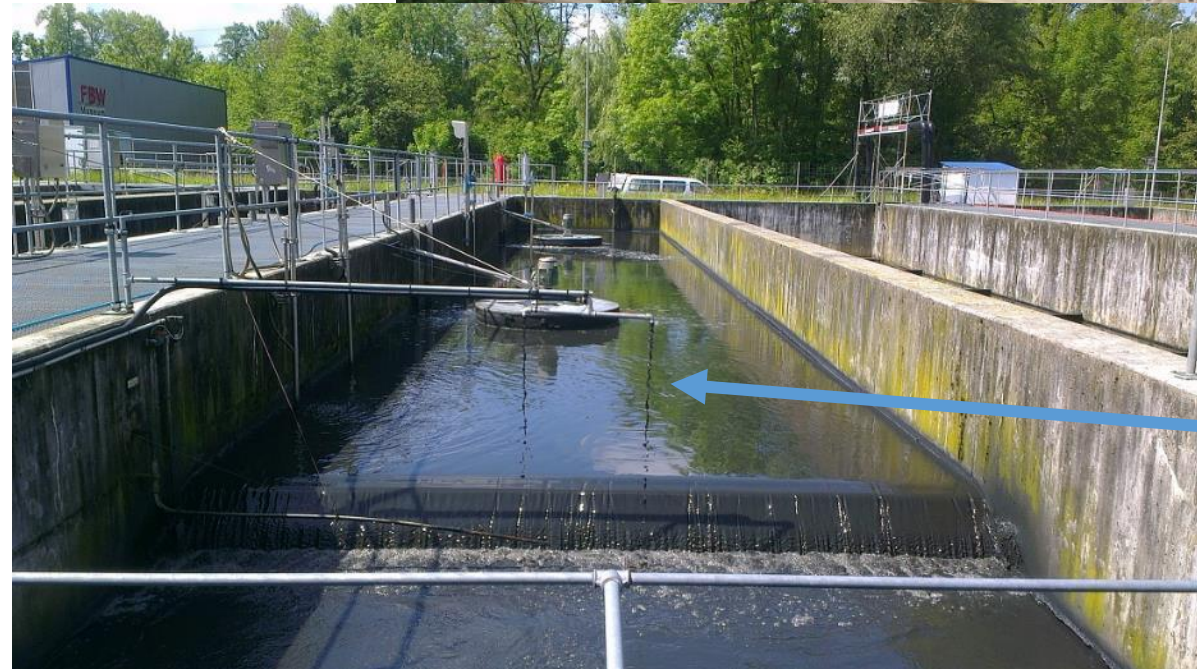
PAC dosage directly into biological tank
